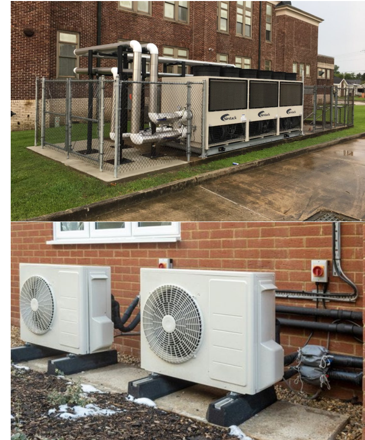
ASHP (top), Split System (Bottom)
