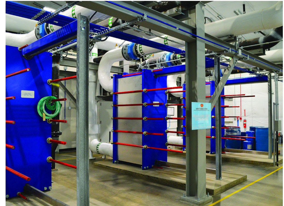
Large Capacity Heat Exchanger
