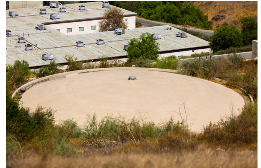
Thermal Energy Storage Tank
