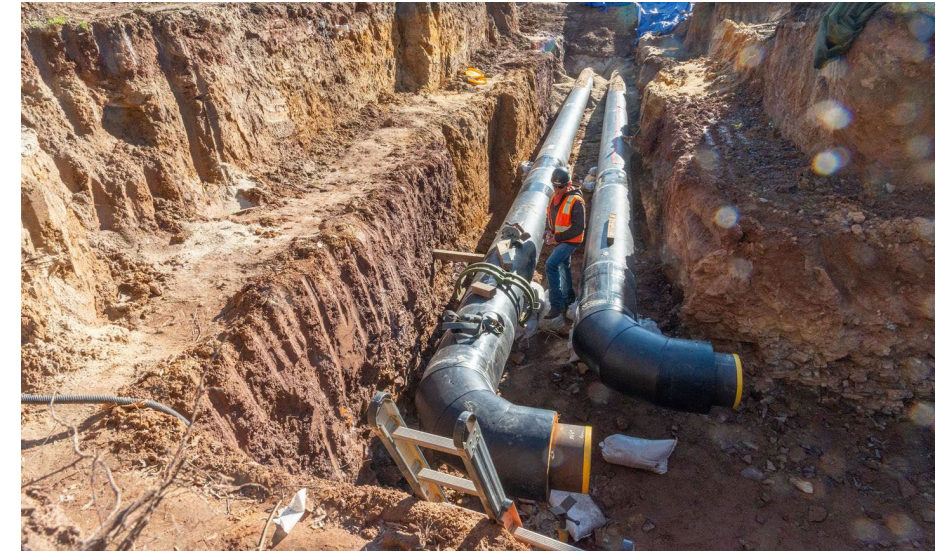
Steam to hot water conversion at Princeton
