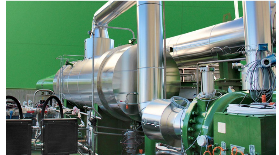
Steam Heat Pump
